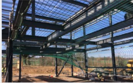
Safety netting – fall arrest system
