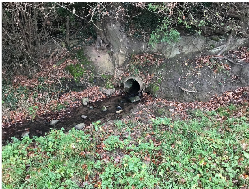
Figure 3: image facing to the south (upstream) of the watercourse as it emerges from a culvert passing beneath a finger of land extending into the site along the eastern boundary.
